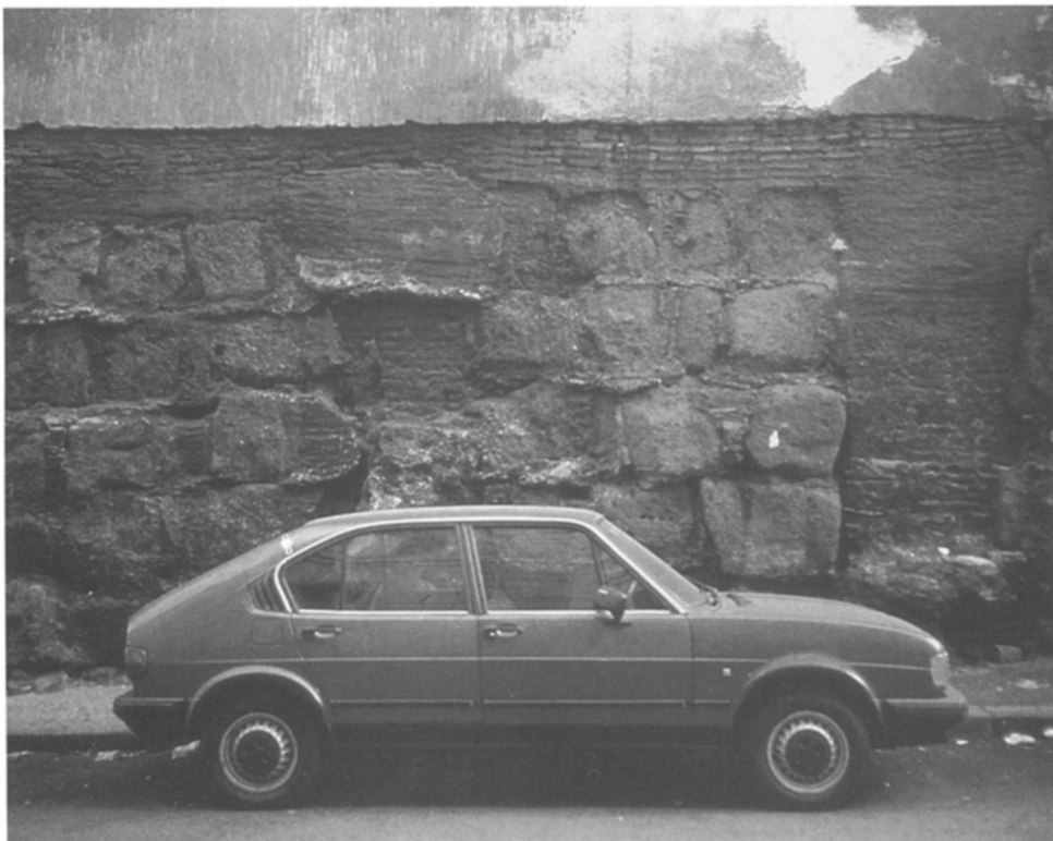
2 SAN MARTINO AI MONTI. EXTERNAL RIGHT AISLE WALL: MASONRY OF RE-USED OPUS QUADRATUM AND BRICK.
