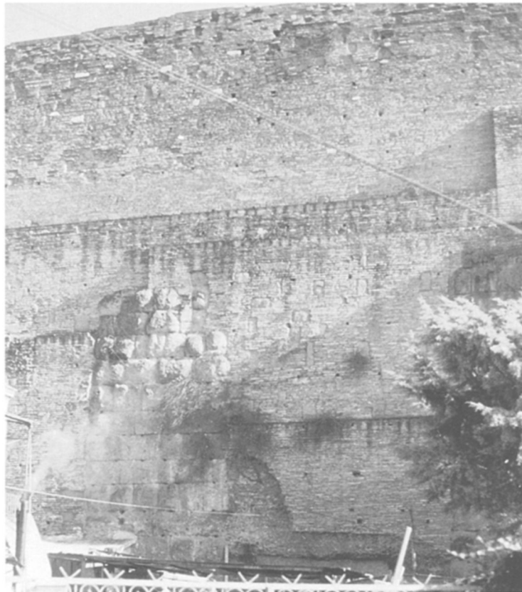
2. AQUA CLAUDIA AT PORTA FURBA. BUTTRESS IN RE-USED BRICK AND TUFA BLOCKS.
